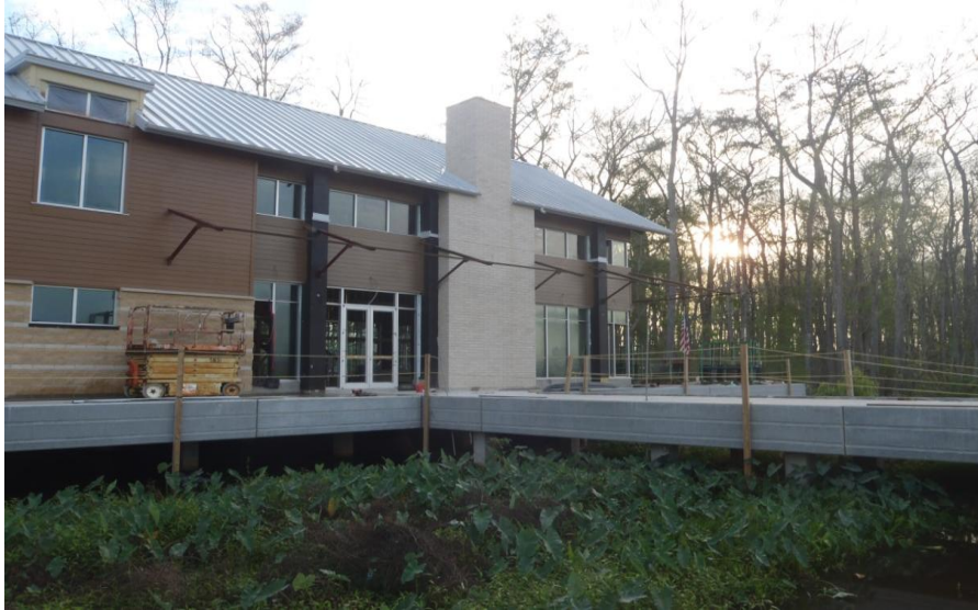
Figure 10. Construction of the Cajun Coast Tourism Center is underway in St. Mary Parish.
